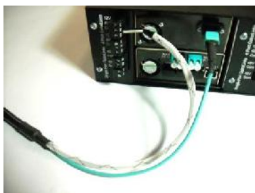
MTP & bare copper conductors connect to rear of a Power Patch Panel
